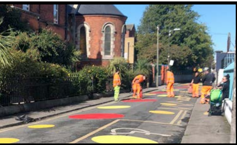
Work is already happening on our 'School Zone', helping keep us all safer.
